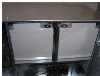
Figure 3 - 24 Vdc monoblocs series installation
