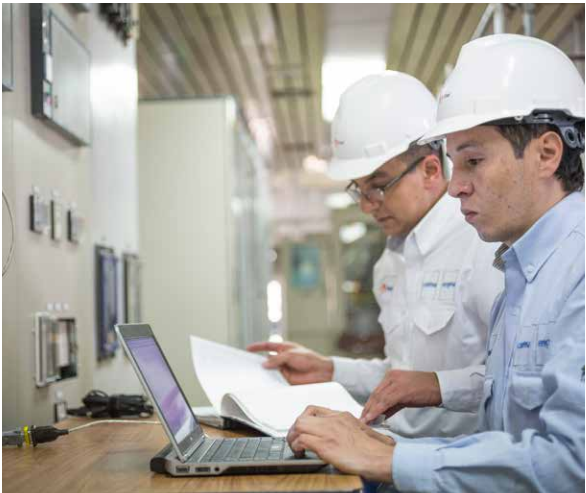
Muña Pumping Station
