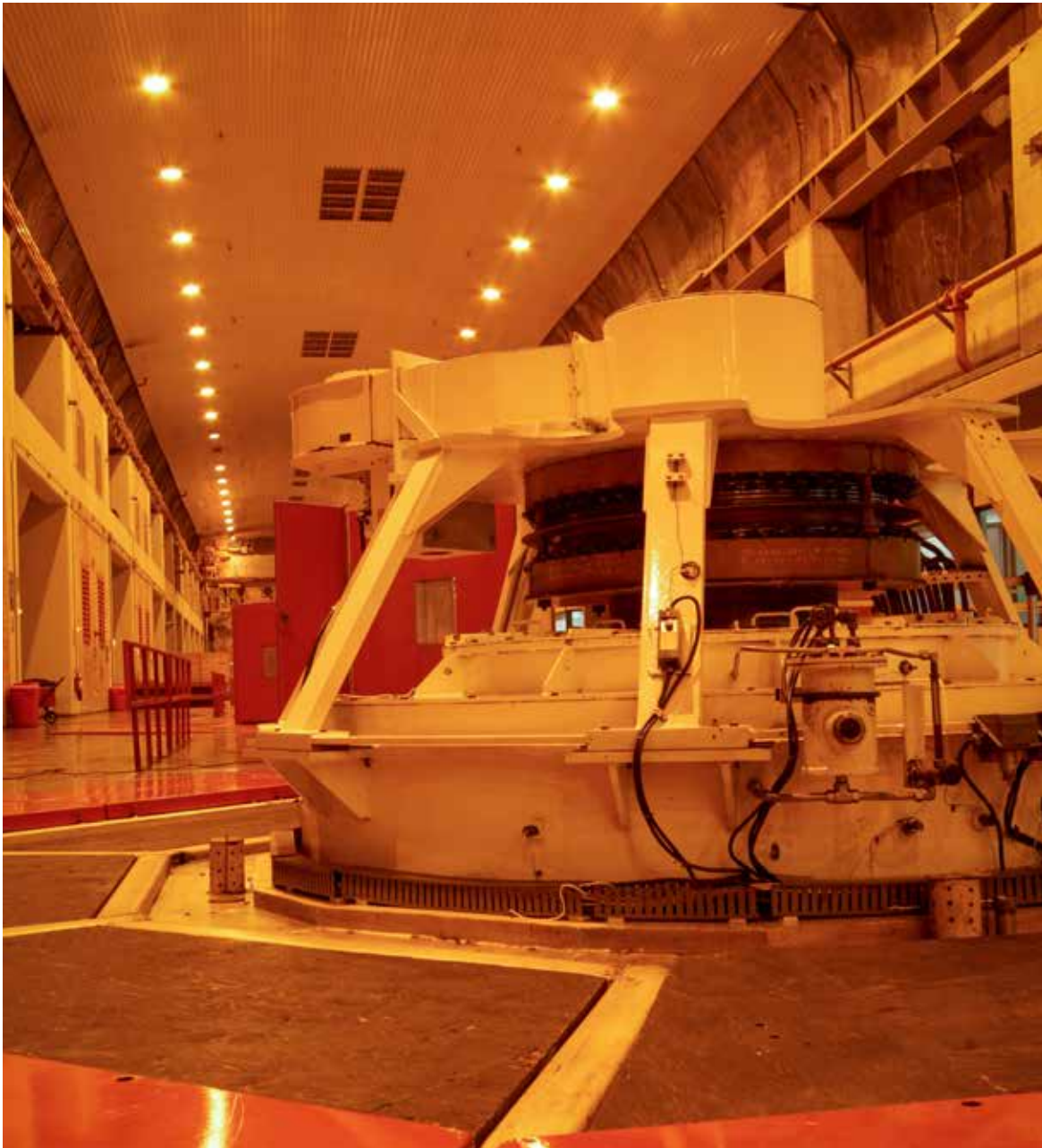
Guavio hydroelectric station
