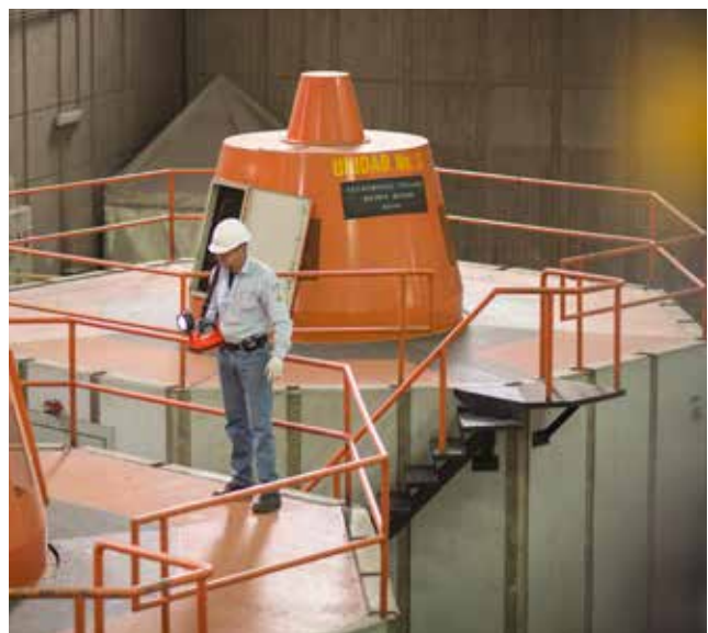
Muña Pumping station
