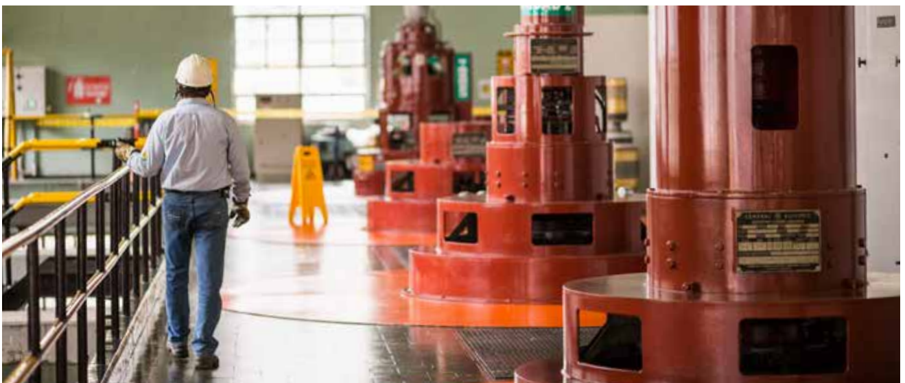
Limonar hydroelectric station
