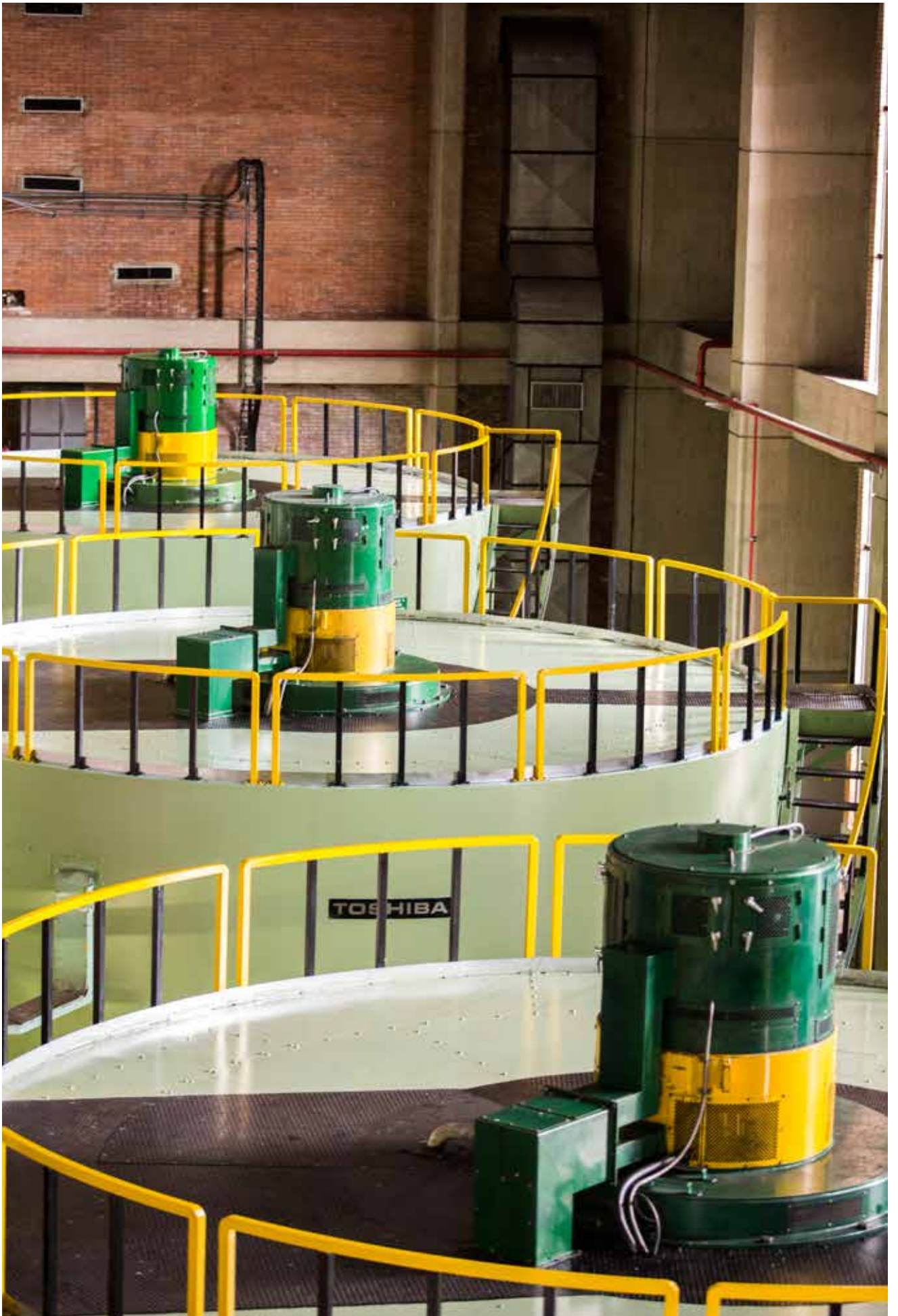
El Paraiso hydroelectric station
