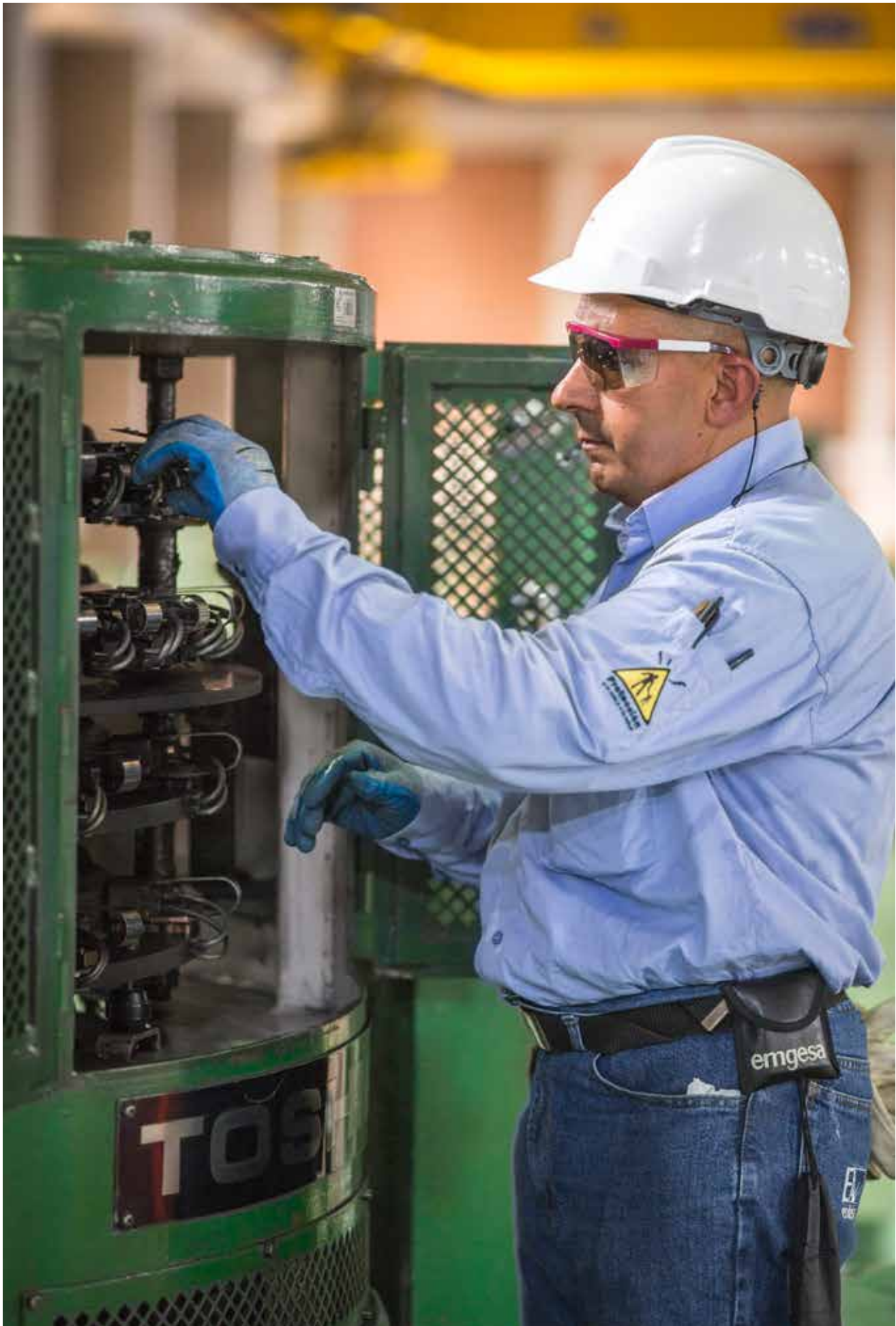
La Guaca hydroelectric station
